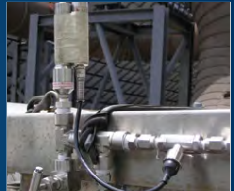
Orifice Plate Monitoring
